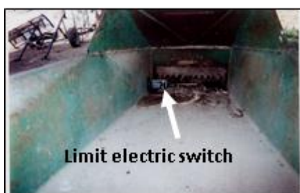
Figure 6. The limit electric switch
