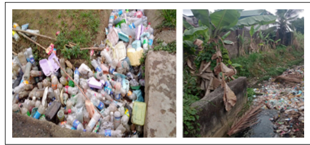
Figure 1. PET/PS blocked drains.
