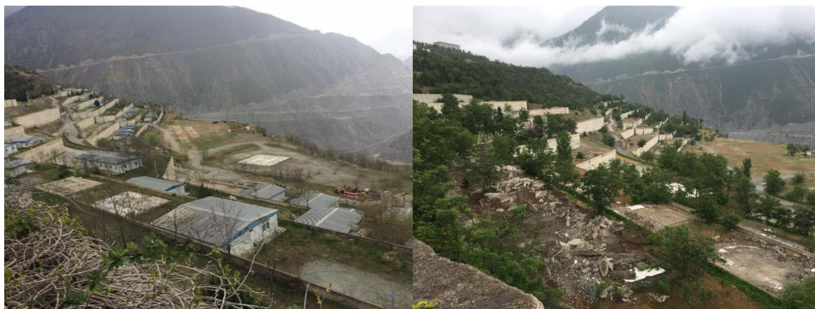
2. The construction site of the area before the botanical garden (May 2005- June 2018)
