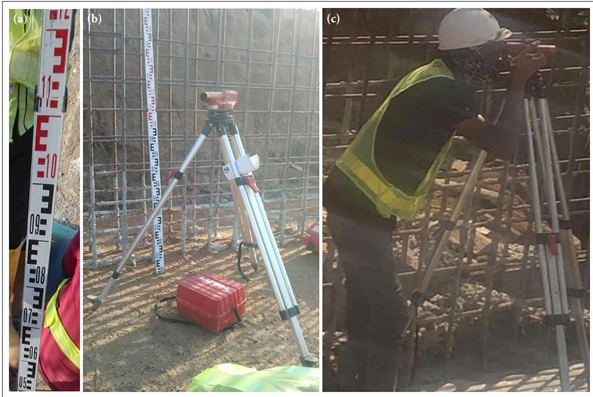
Figure 4. (a) Survey Staff (b) Level device fixed on tripod stand (c) Taking of road levels by the chief surveyor.
