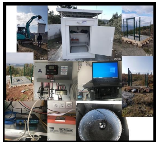
Figure 2. Instruments of the DEUNET seismic network (station installation).
