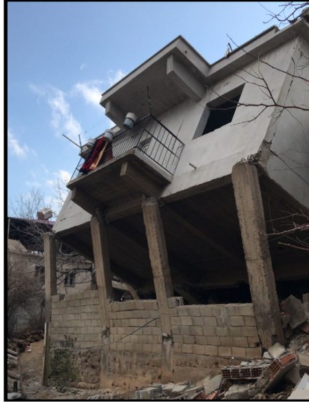
Şekil 7: Zayıf kat sonucu hasar alan bina örneği, Hatay (TMMOB MO ve İMO İzmir Şb. 2023) Figure 7: Example of a building damaged by a weak floor, Hatay (TMMOB MO and İMO İzmir Br. 2023)
