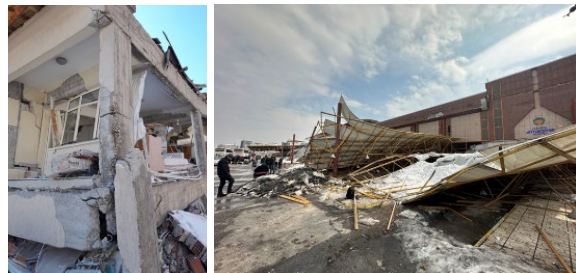
Figure Damage assessment of reinforced concrete and steel structures
