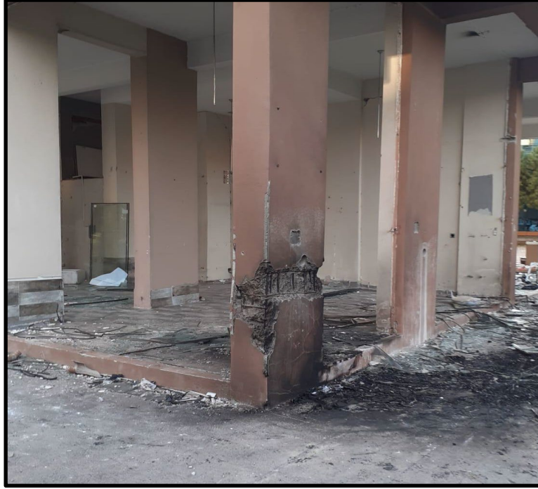
Şekil 30: Deprem sonucu hasar alan zemin kattaki kolon (Çetiner 2022) Figure 30: Column on the ground floor damaged by the earthquake (Çetiner 2022)
