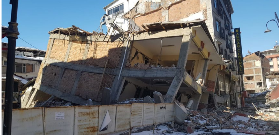
Şekil 10: Zayıf ve yumuşak kat nedeniyle hasar alan bina Figure 10: Building damaged due to weak and soft storey
