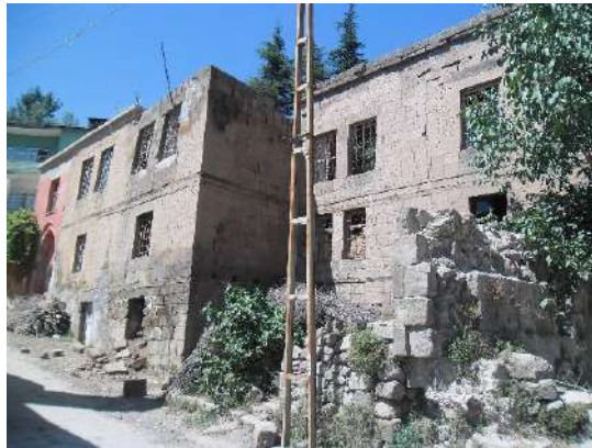
Figure 3. Zeydan neighbourhood, block 498 parcel 5, 6, rectangular double window row on the 1 st floor façade (source: author, 2013)
