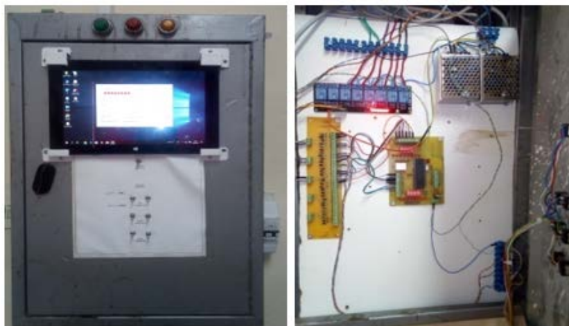
Figure 12. Internal and external view of the system
