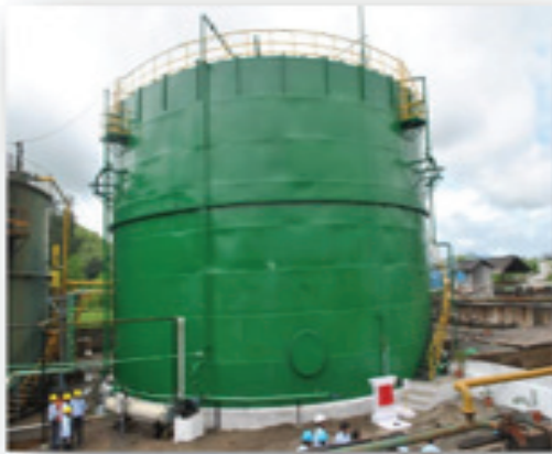
(a) Fixed Film Digester for Pharmaceutical Effluent, Embio Ltd. India
