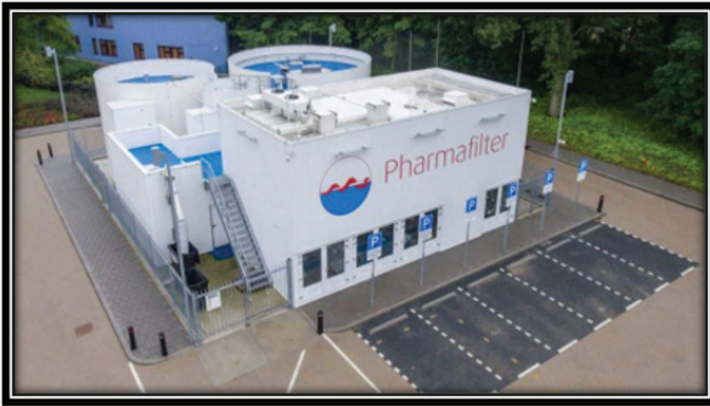
Figure 5. Anaerobic digestion of hospital waste in Amsterdam, Netherland. [From Burik [213], with permission from LABIOTECH].
