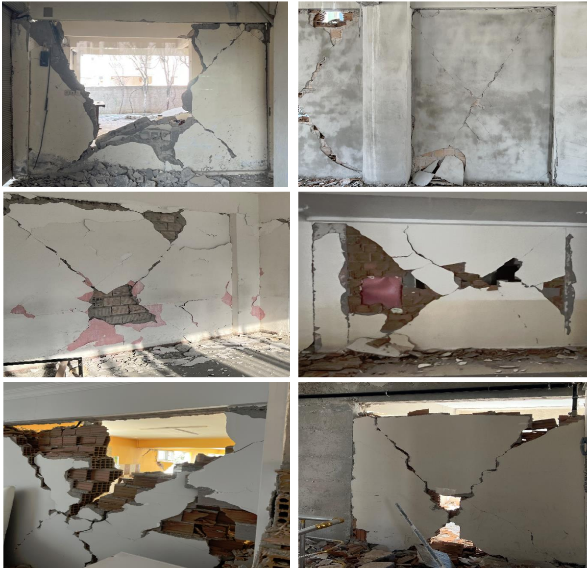
Figure 1. Diagonal cracks in infill walls after Kahramanmaras earthquakes.
