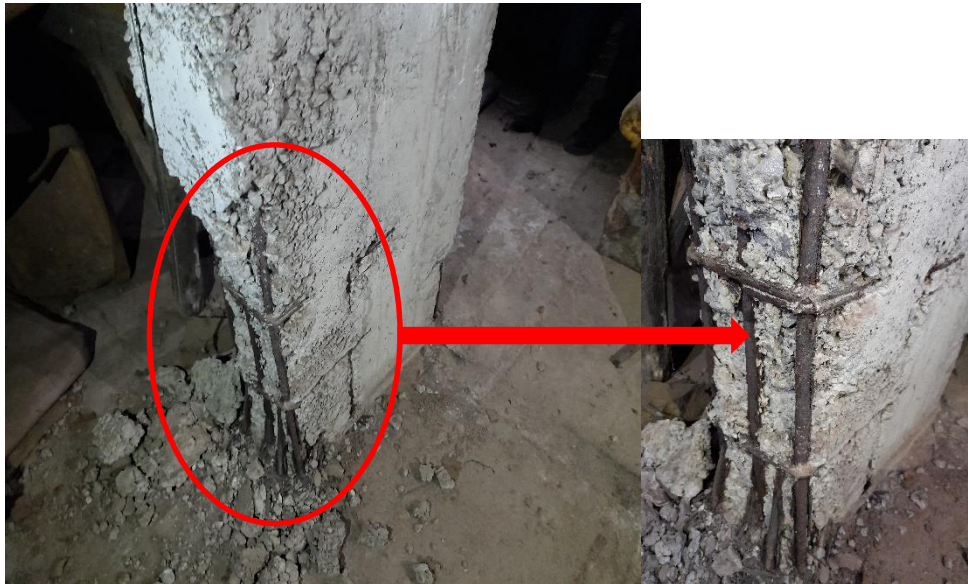
Figure 4. Crust loss in the column and corrosion in the reinforcement
