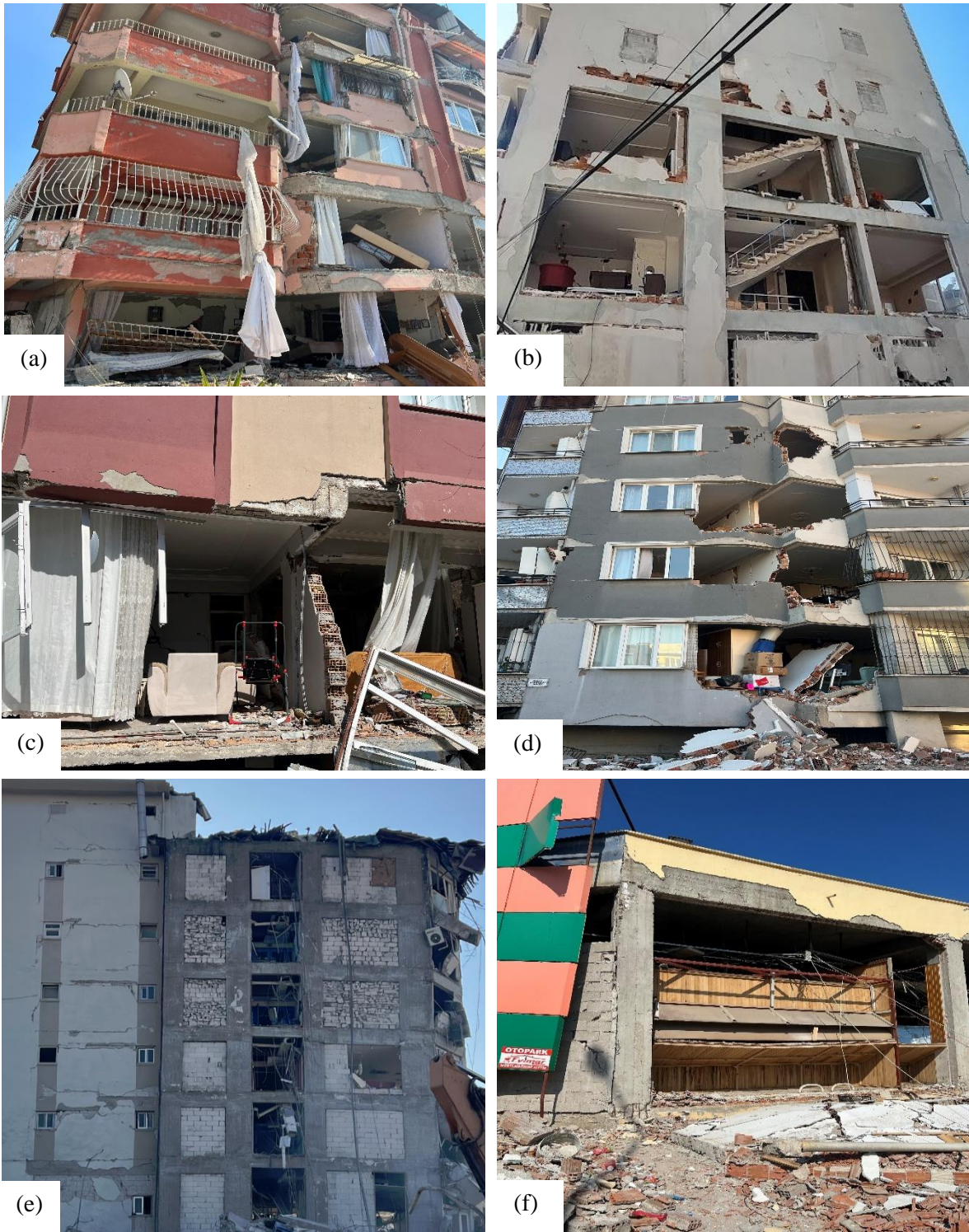
Figure 2. Out-of-plane behavior in the infill walls occurred after the Kahramanmaraş earthquakes, (a), (b), (c), (d) brick infill walls, (e) aerated concrete infill wall and (f) briquette infill wall.
