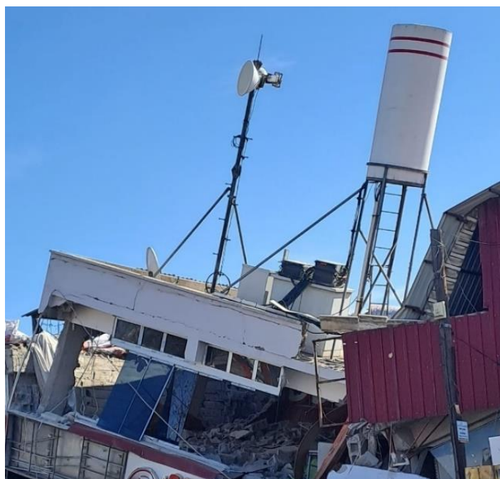
Figure 3. Roof-top Base Stations under Disaster Effect
