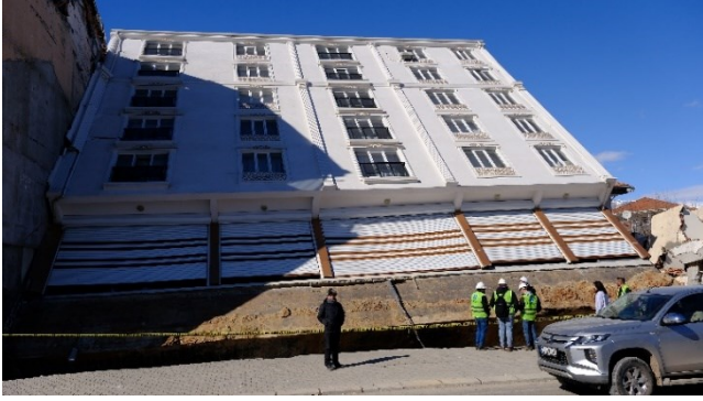
Figure 1. A building that collapsed due to soil liquefaction but remained intact based on its elements.
