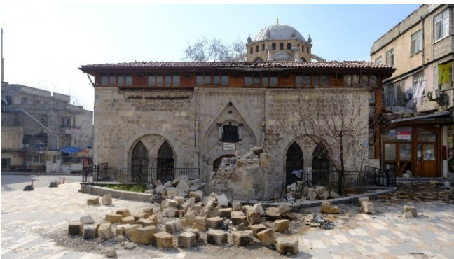
Figure 7. The Historical Arasa Mosque in the Kahramanmaraş earthquakes
