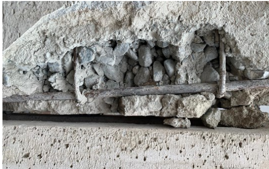
Figure 17. It is seen that the concrete was placed with segregation and without a vibrator.
