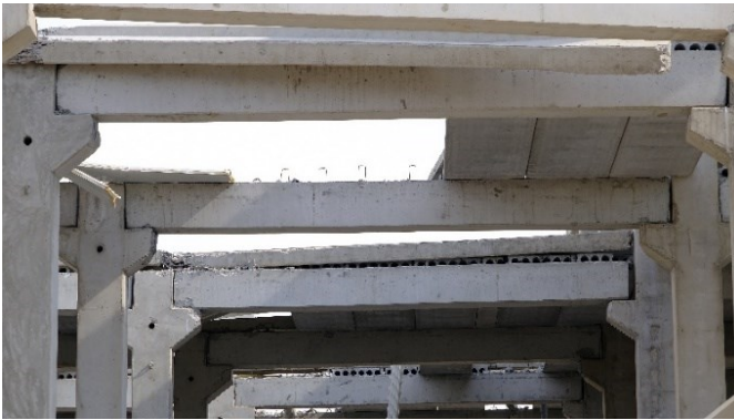
Figure 10. Damage occurring at the connection points of the prefabricated structure
