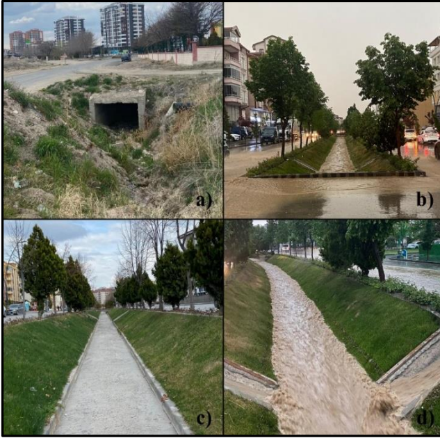
Figure 3. Culvert inlet (a), outlet (b) and open channel downstream of the culvert (c, d)
