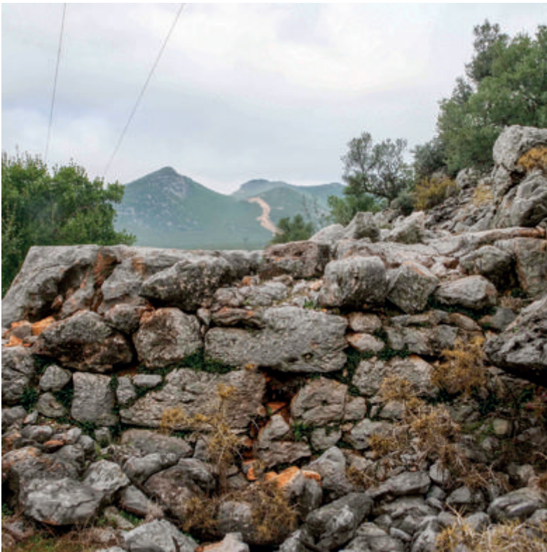
FIG. 6 Döşeme Boğazı. Upper site. "Northern boundary wall." Interior face. View from south.
