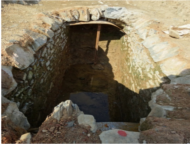
Figure 7: Damaged vault from the original phase of the aqueduct channel.
