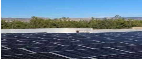
Figure 4. CIU block b roof solar installation.
