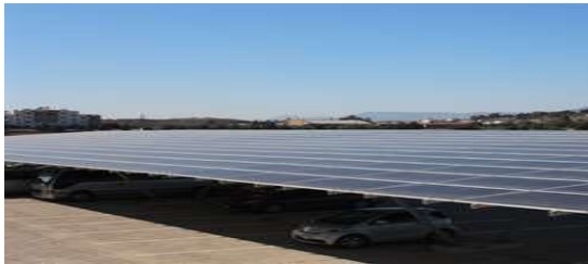
Figure 5. CIU arena solar installation.
