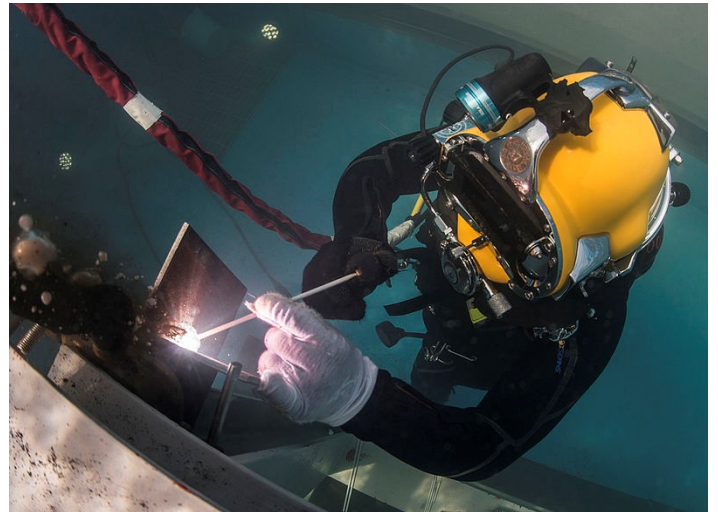
Fig. 4. JINHAE, Republic of Korea (March 15, 2016) U.S. Navy Builder 2nd Class Jesus Saucedo Gomez (right) with Underwater Construction Team (UCT) 2, performs an underwater fillet weld in a training pool at the ROK engineering school at Jinhae, ROK during exercise Foal Eagle 2016. Foal Eagle is an annual, bilateral training exercise designed to enhance the readiness of U.S. and ROK forces, and their ability to work together during a crisis.
