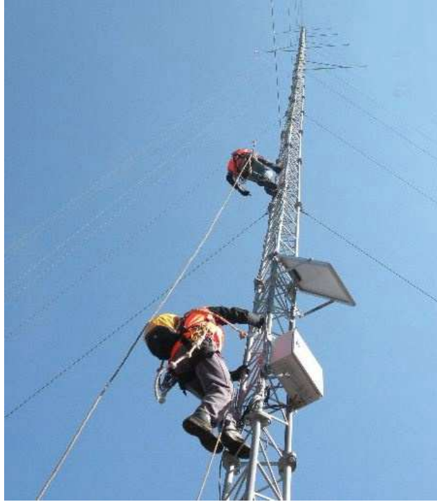
Photo 1. Wind Measurement Pole and Equipment(WOS).
