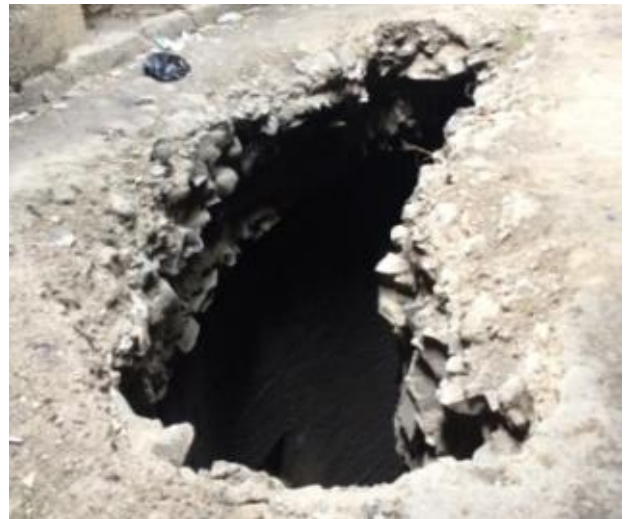
Figure 9. Slit formation on Tower 20' due to the slumps
