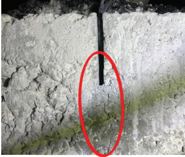
Figure 16 - Dual wheel induced cracks under the unreinforced contraction joint
