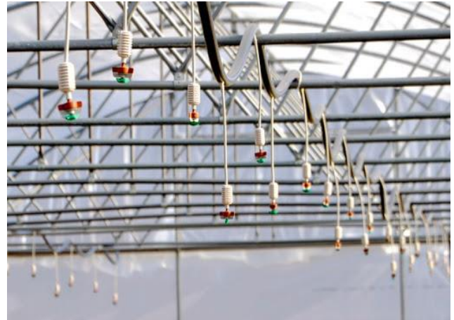
Fig.3. Greenhouse sprinkler systems
