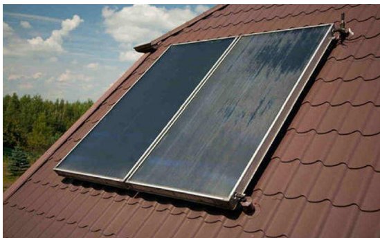
Figure 1.3. Flat Plate Solar Collectors [20]
