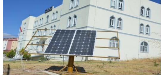
Figure 8. Solar Tracking System
