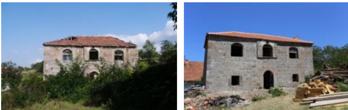
Figure 11. Kulla of Sali Kajtazi in Kqiq Village, Kosovo, listed on Heritage at Risk Register (Left: in a very bad physical condition, right: improvement of the condition by the Ministry of Culture) (By author, 2016 and 2017)
