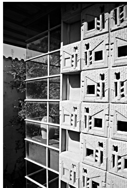
Fig.8: Textile Block construction system, c.1922. Fig.9: Corner detail from Samuel Freeman House (1923, Hollywood Hills, LA).
