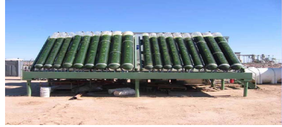
Figure 15. Algaepower GmbH Manhattan, A newly installed photobioreactor in the USA
