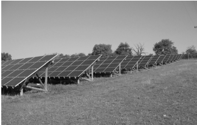
Figure 2. The PV power plant Bušanovice
