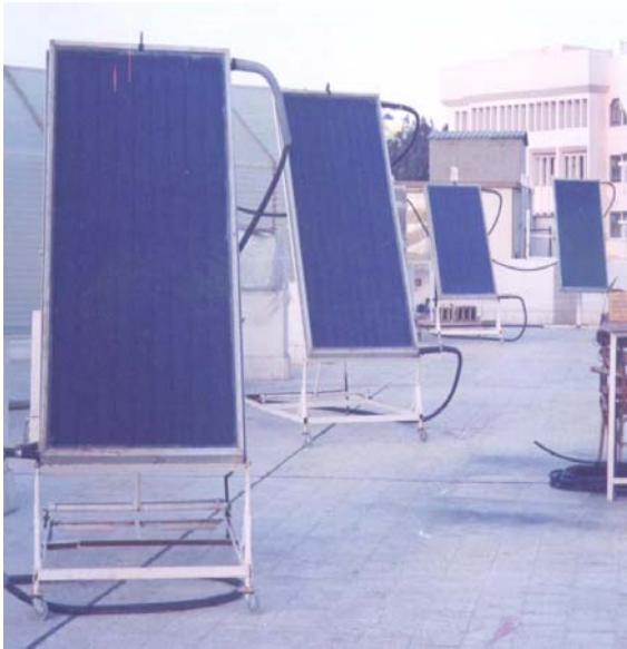
Fig. 1. Solar water heaters during operating the heating system.
