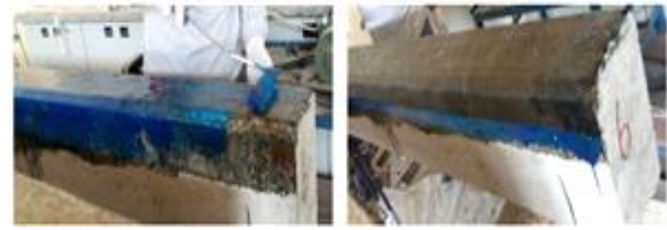
Figure 2. CFRP application of test beams a) epoxy adhesive application b) bonding of CFRP
