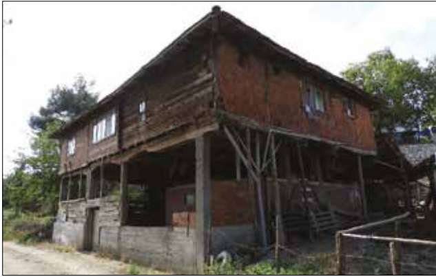
Fotoğraf 59. Ahşap dikmeler yerine betonarme ayaklar, Salar Köyü, 2018 / Reinforced concrete pillars instead of wooden posts, Salar Village, 2018.
