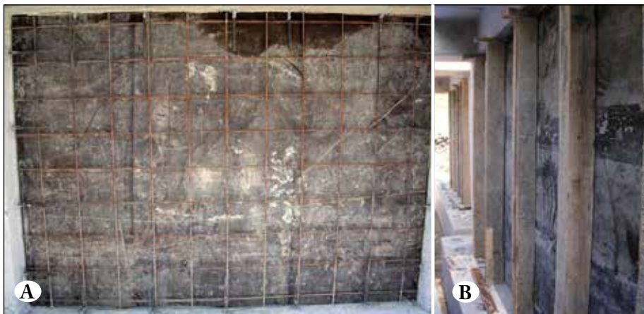
Figure 2. Construction of the shotcrete panels. A) Wire mesh and one layer of formwork. B) Back view of formwork.
