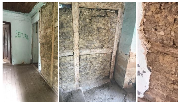
Figure 6. Visible wall structure of the Pozderac family house in Cazin (Ahmet Hadrovic, 2019)
