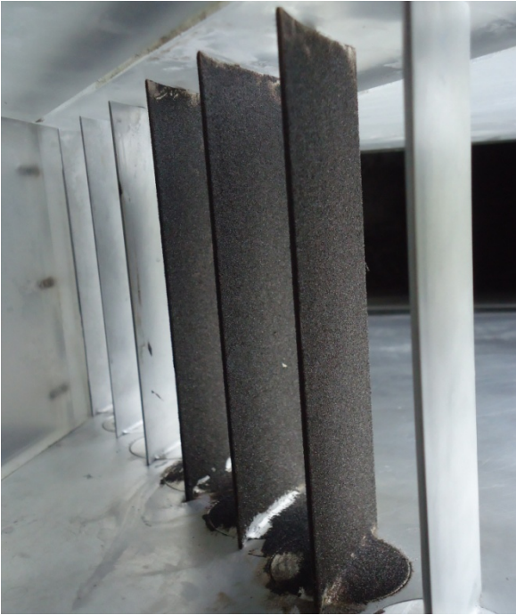
Figure 7: Fouled and Washed Blades
