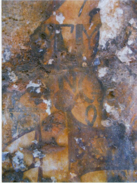
Fig.13 - The letter remains on the second cross arm of the south wall.
