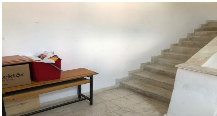
Figure 1. The obstacle in the Fire Escape and Not Using Anti-Slip Tapes
