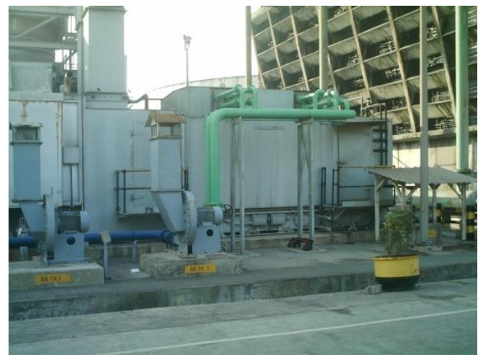
Fig. 1. Gas Turbine Generator (GTG) at PT. PKG
