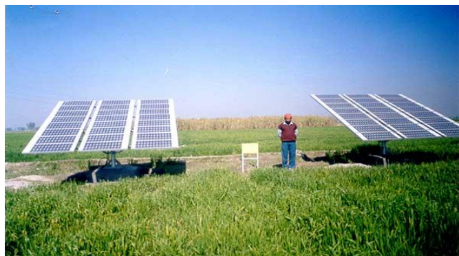
Fig. 10. A solar water pump installed in a village in Punjab
