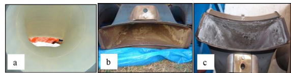
Figure 10. Visual inspection of transition piece (a) before operated (b) after operated by HSD taken on Major Overhaul (c) after operated with B5 for 1 month
