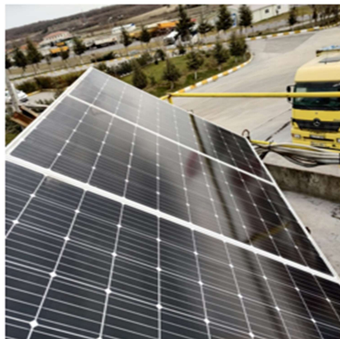
Figure 5. PV panels in the system
