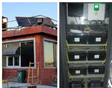
Figure 3. The installed system
