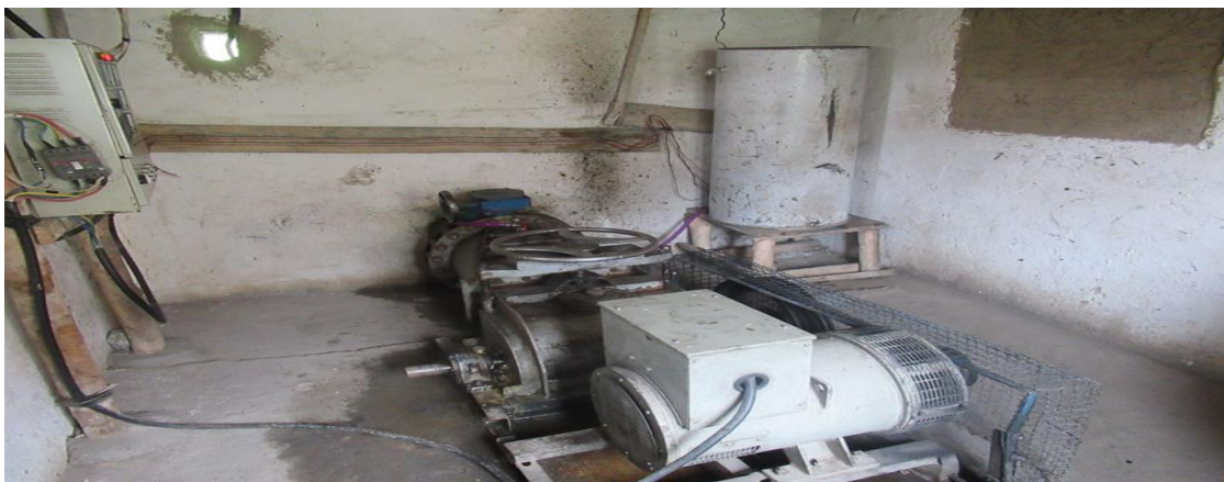
Picture 2: Turbine of one of Micro-hydro Power Plants- Badakhshan Province –Afghanistan
