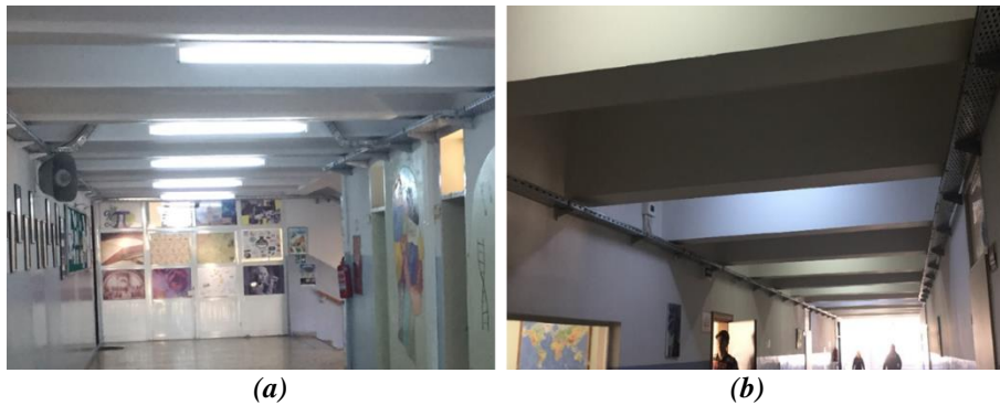
Figure 5. Location of lighting armatures: (a) 1st-floor corridor, (b) Ground floor corridor.
