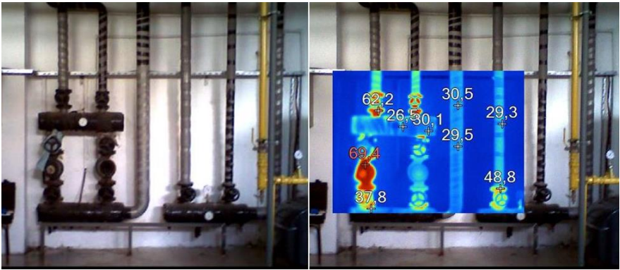
Figure 10. Thermal images of the heating installation in operating conditions.
