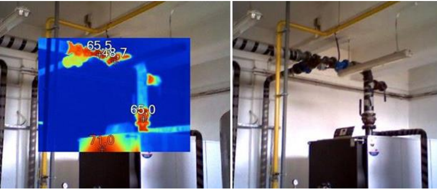
Figure 11. Thermal images of uninsulated valves.
