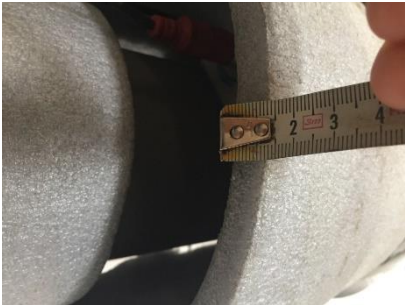
Figure 9. Insulation material and application thickness used in the heating system pipeline.
