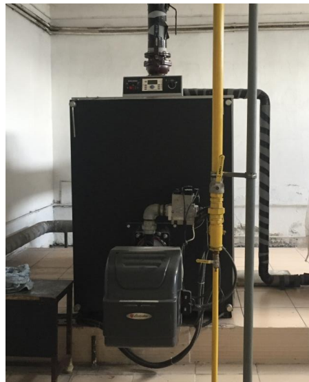
Figure 2. Existing hot water boiler.
