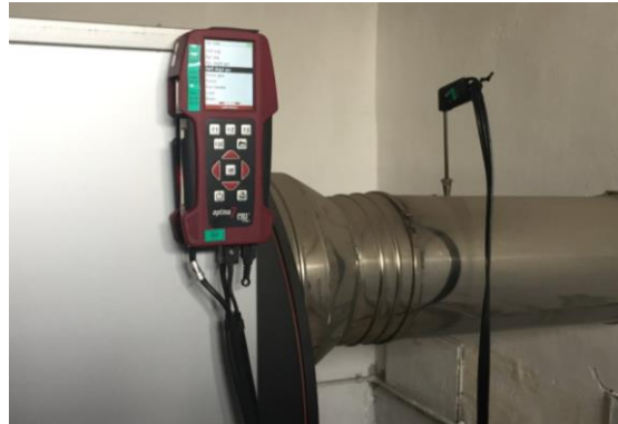
Figure 3. Flue gas analysis probe connection point.
