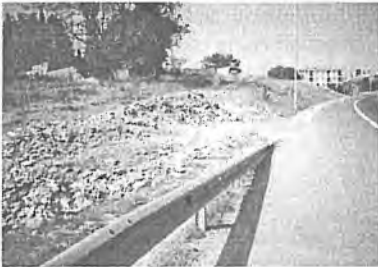
Şekil 8 : Otoyol şevine dökülmüş moloz Figure 8: Stones and soil material on the
