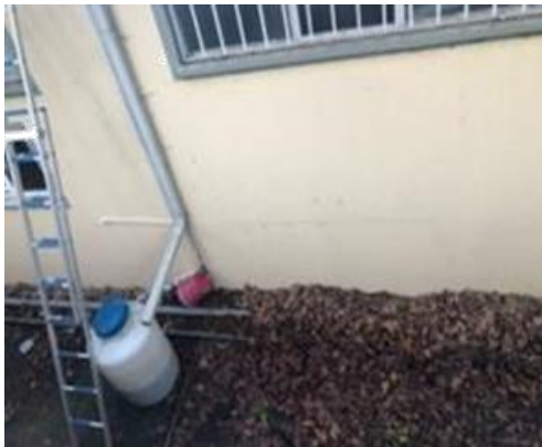
Figure 9 Water tank and pipes
