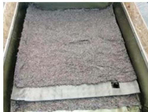
Figure 6 The third geotextile felt moisture trap placed on the root retaining layer
