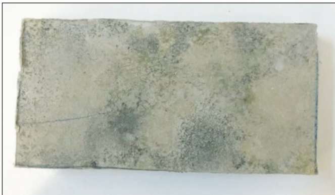
Figure 3. Dark mould fungi on the surface of plasterboard.
