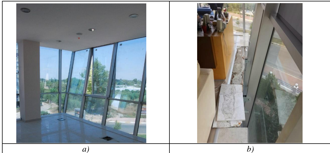
Figure 3. Photographs of GCW system from interior figure; a) View of the GCW from the interior ample b) Detailing of the GCW which leads to heat exchange between the floors
