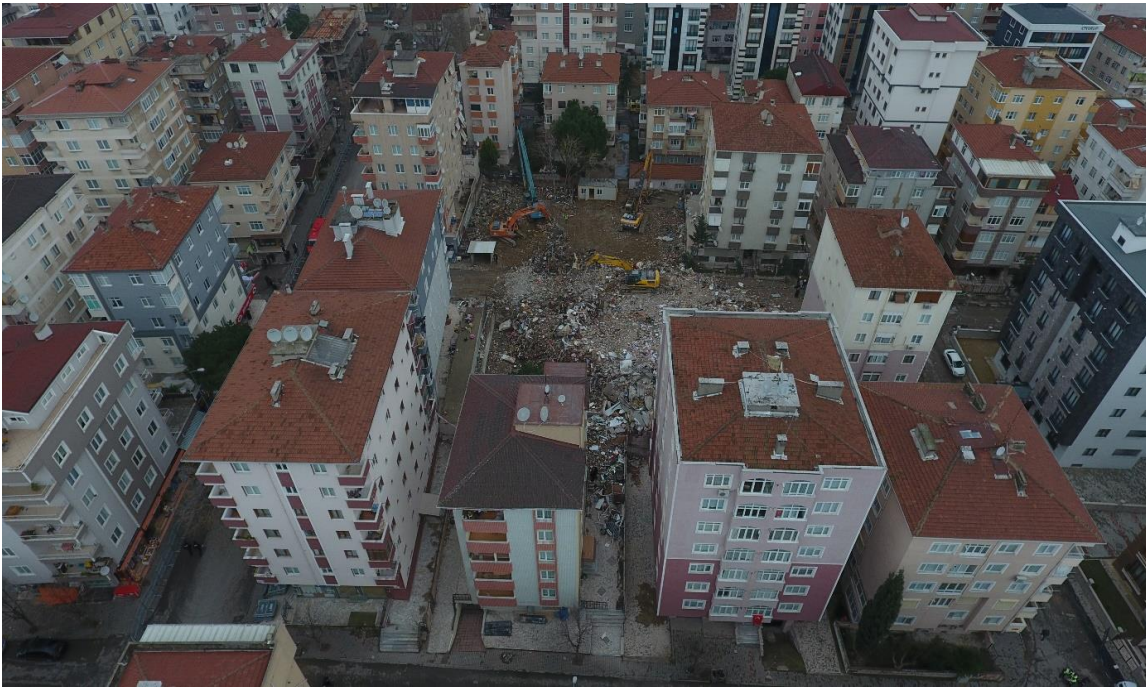
Figure 11. The View After Removal of The Wreckage of Yeşilyurt Apartments
