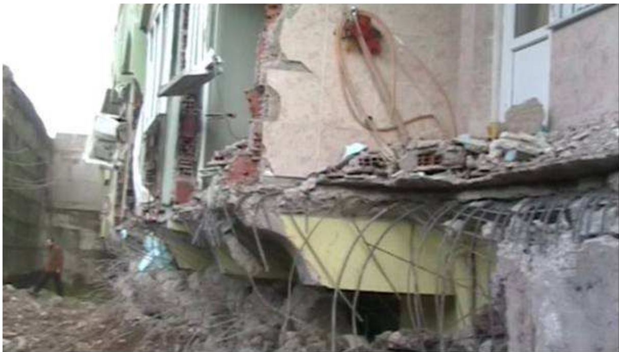
Fig. 3. Severe damage of the building knocked by the retaining wall
