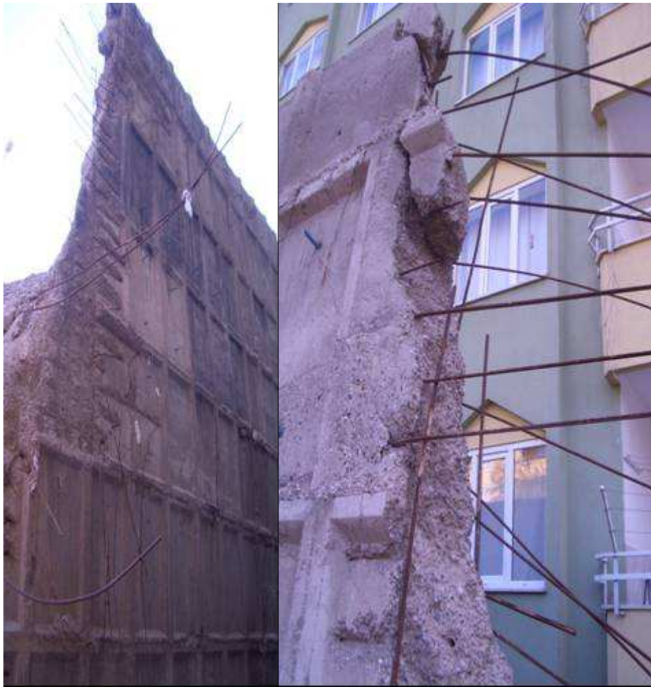
Fig. 2. Collapsed retaining wall
