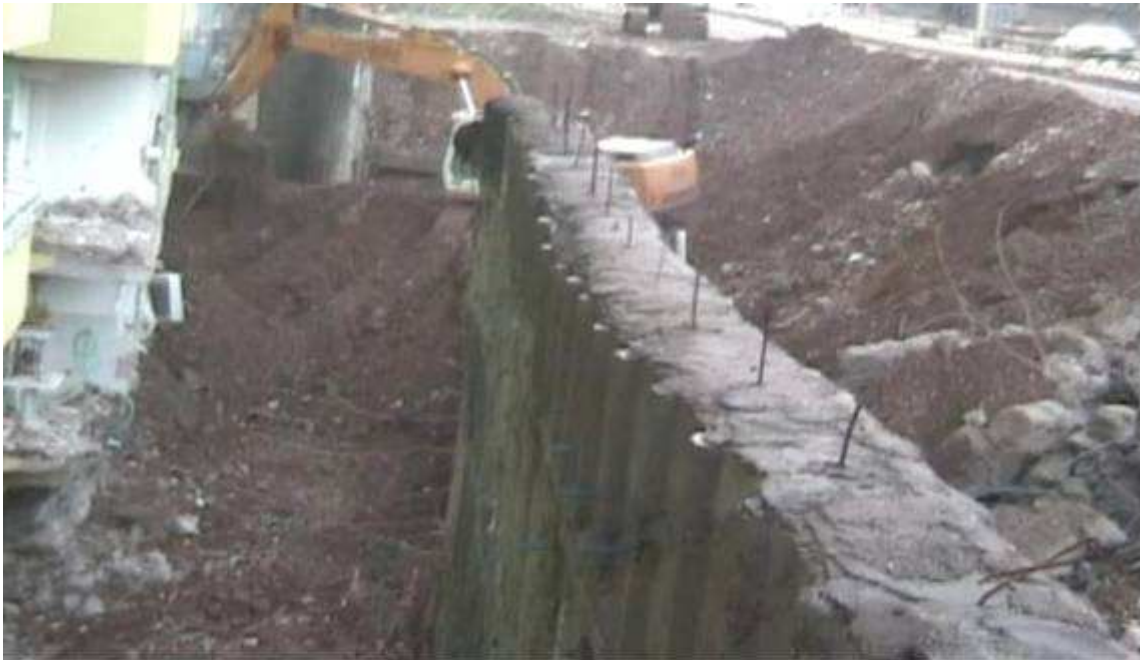
Fig. 1. Retaining wall failure
