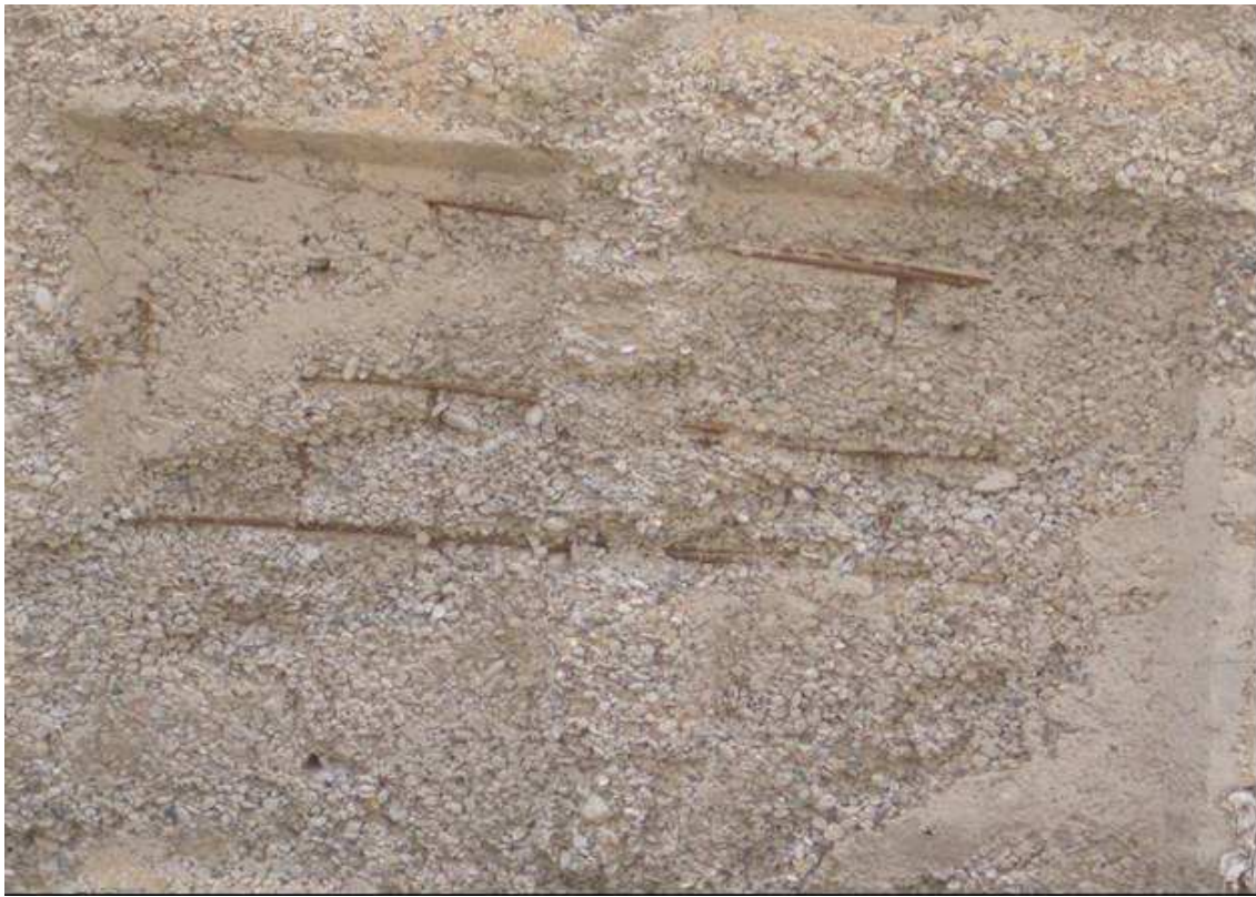
Fig. 5. Segregated concrete of the RW
