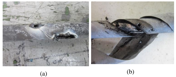
Figure 3 The Structural View of cable after test operations; a) 250V applied state, b) 500V applied state
