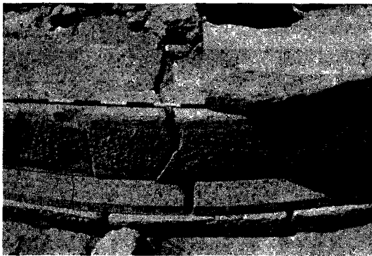
Fig. 68 — Northeast section of podium showing crack
