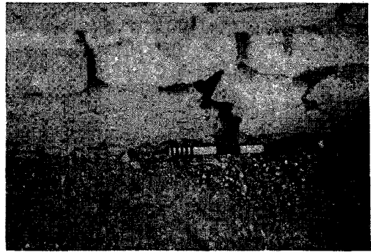
Fig. 69 — Wall of Byzantine structure to the north east of the podium displaying a crack in the wall, southwest to northeast.
