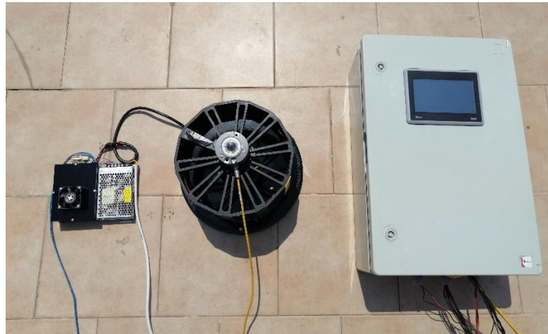
Figure 7. The experimental setup consisting of RES, controller and PLC measuring station
