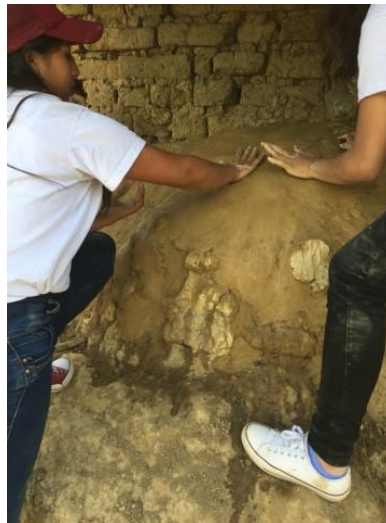
Figure 1. Application of soil plasters stabilized with Opuntia mucilage in a historic furnace, during a restoration training workshop in Villa de Leyva, Colombia (Photo: L. Guerrero).
